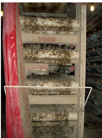
Figure 3. Cross-conveyor Belts at Cage Tiers Ends.
